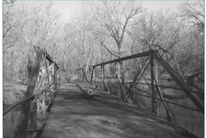
74B-012 Queen Anne Bridge Patuxent River at Queen Anne Bridge Road Queen Anne
