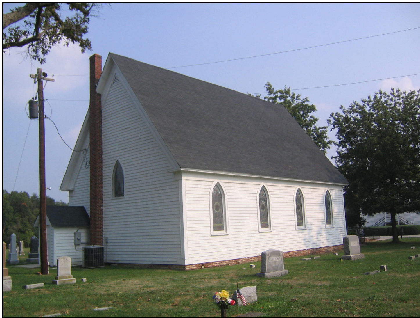
Photo: Immanuel Methodist Church, view of the west (side) elevation, looking southeast. (August 2007)
