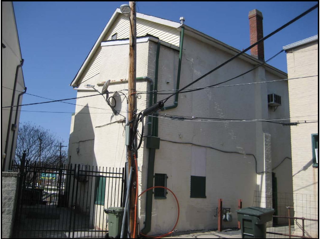
Photo: Potts/Star Hall, Mount Rainier, view of the southeast (rear) elevation, looking northwest. (March 2010)
