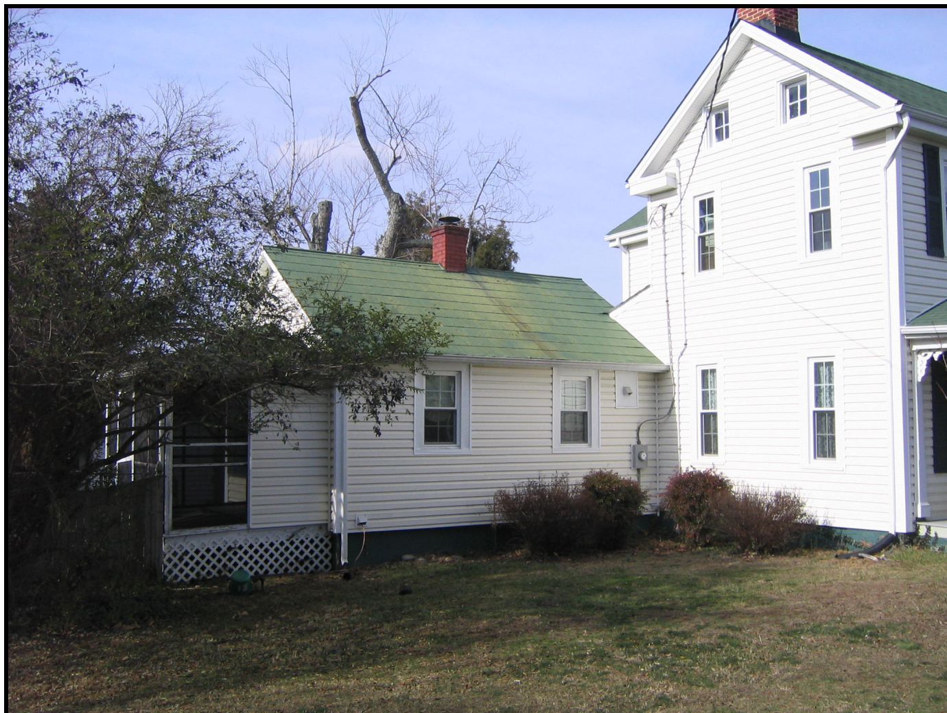
Photo: Mary C. B. Cochrane House, c. 1875, south (side) addition, looking northwest. (January 2008)
