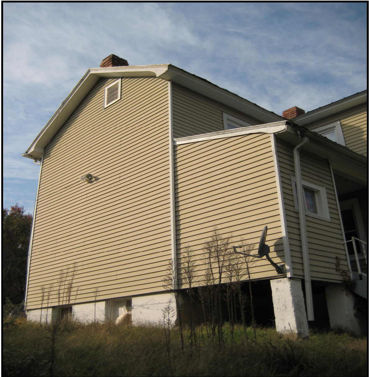
Photo: Proctor House, view of the south (rear) elevation, looking northwest. (November 2007)
