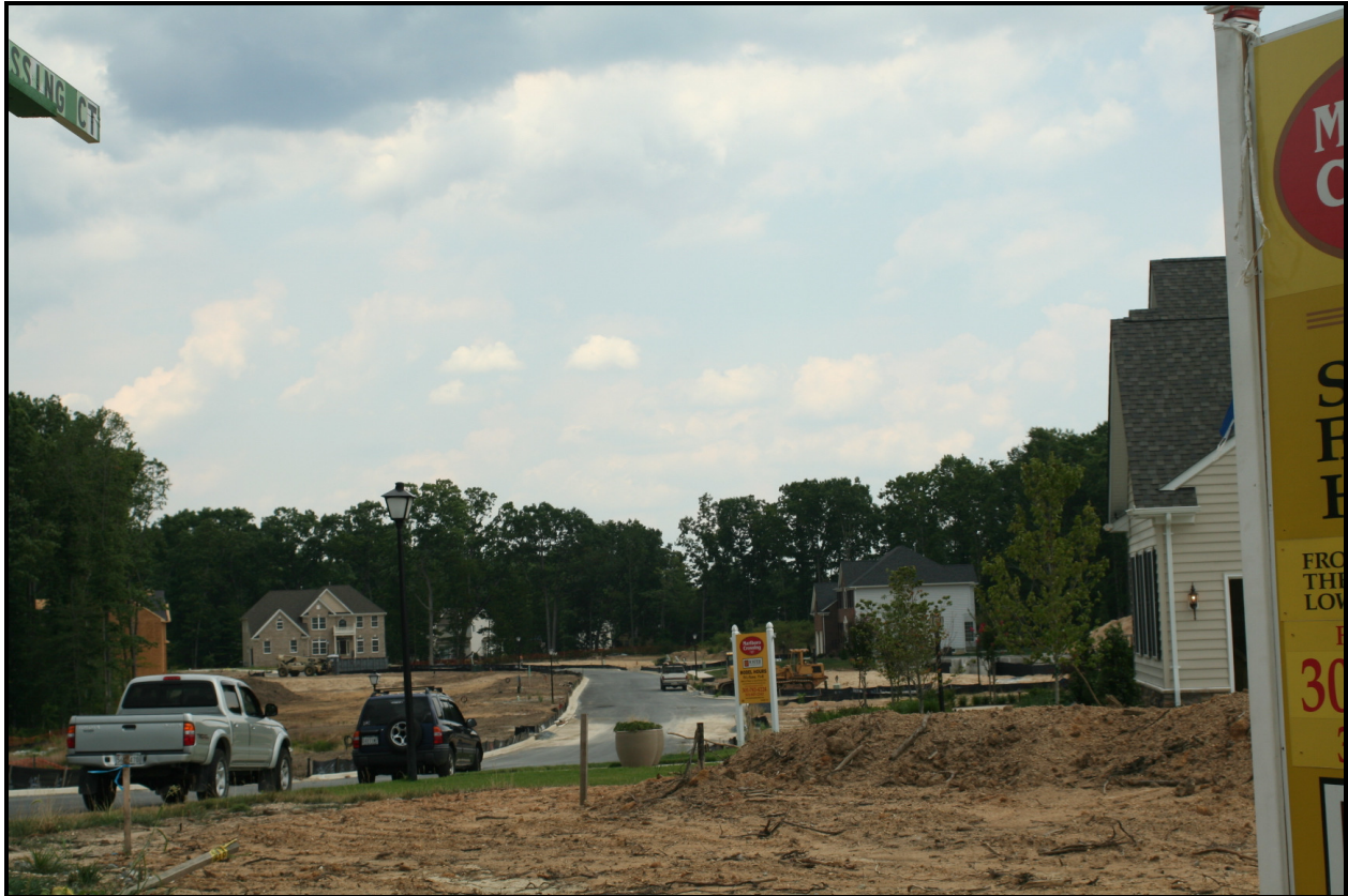
Looking east, Marlboro Crossing Court, part of new Marlboro Crossing subdivision by Foster Homes ( EHT Traceries , 2007)
